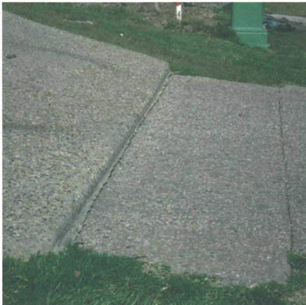
Example of a driveway not joined to crossover
