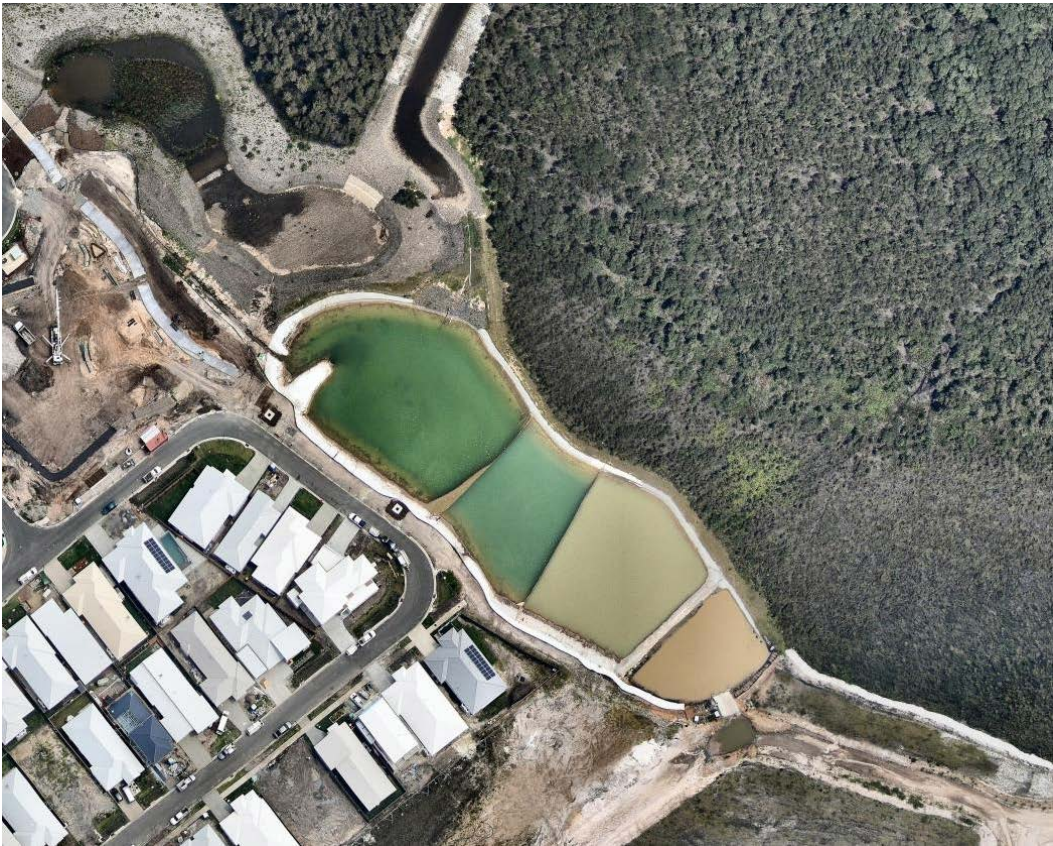
Figure 8: High efficiency sediment basin installed as part of Precinct 2 works – construction runoff treated as it moves through the basin
