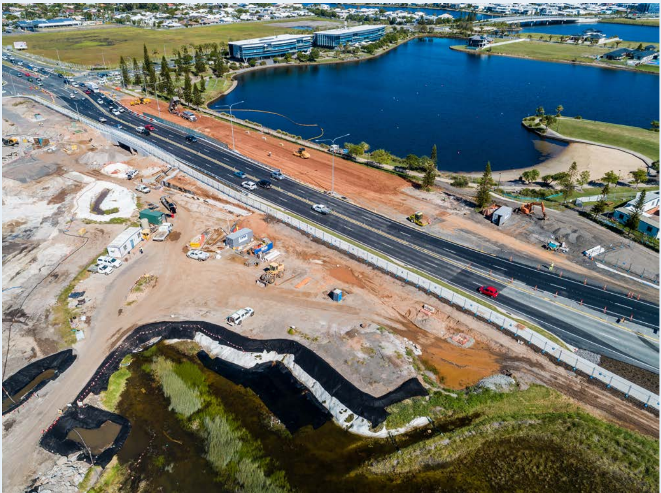
Aerial image of upgrade works at Nicklin Way, adjacent to our Aura (Qld) community.
