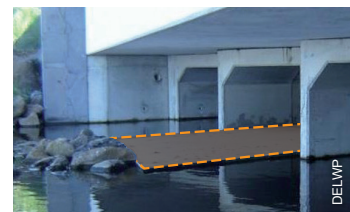
The soil and rock mix will be installed in the base of the culverts
